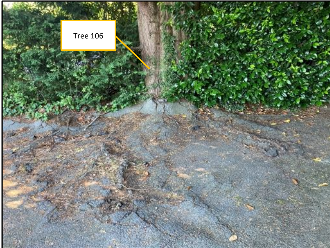
Photo 2. Tree 106 is causing significant damage to the existing driveway.
